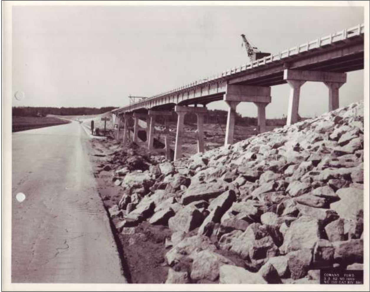
Figure 2.29. Rebuilding North Carolina Highway 150 for its new elevation over Lake Norman, showing old road and bridge (left) and new (right). Photo dated March 1962.
