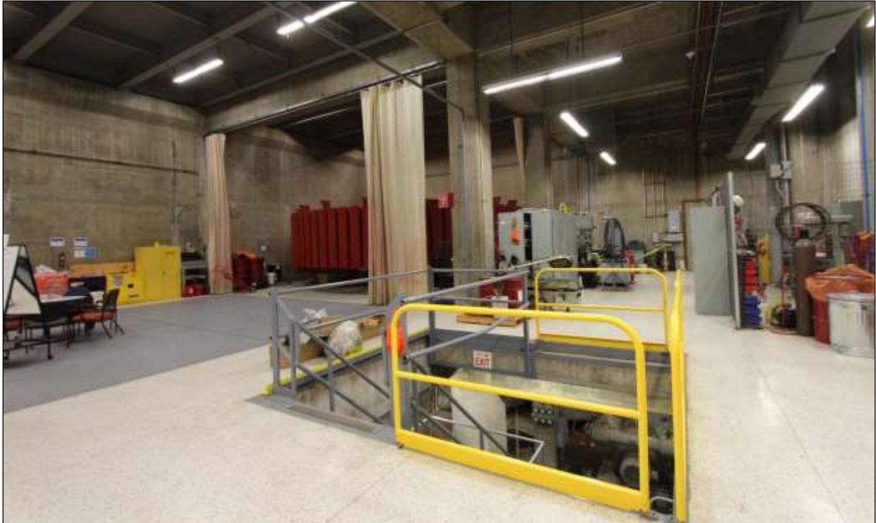
Figure 3.10. Powerhouse interior, service gallery, facing north.
