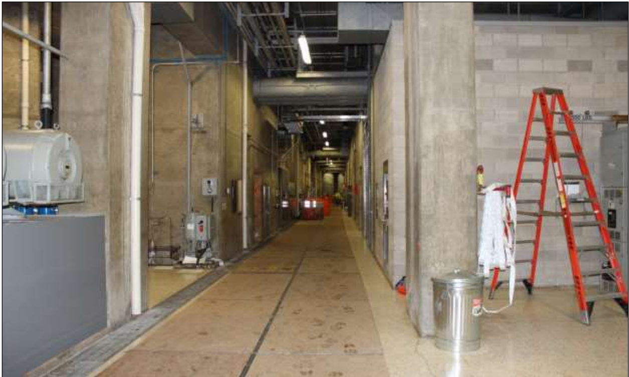
Figure 3.11. Powerhouse interior, gallery adjacent to casings enclosing the generating units, facing east.
