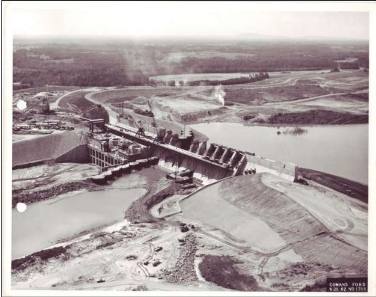
Figure 2.21. Cowans Ford, June 1962, showing progress. The earthen dam (serpentine structure) can be seen just above photo center.
