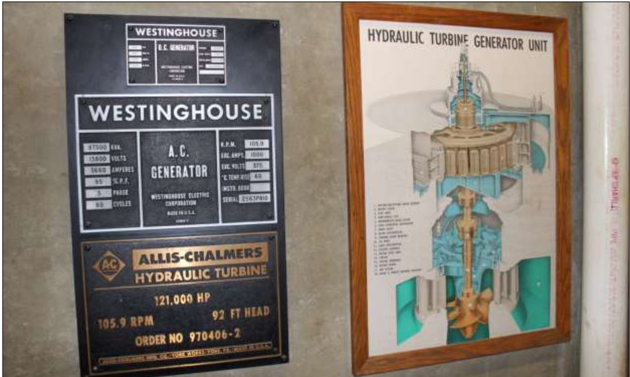
Figure 3.13. Nameplate for generating unit.
