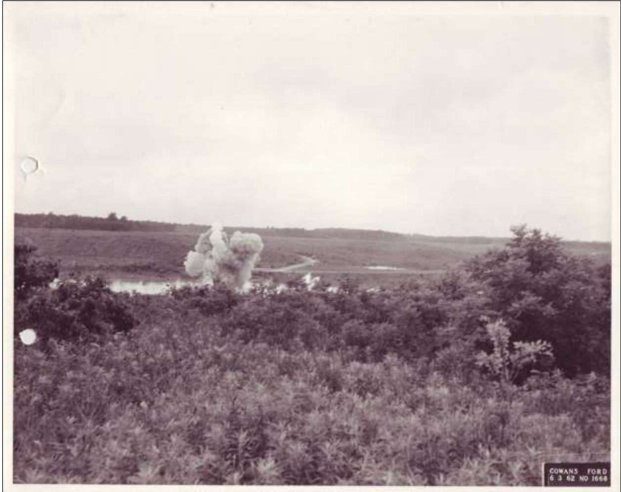
Figure 2.33. The Beattie's Ford Bridge was used as a training exercise for U.S. Army and U.S. Army Reserve demolition units and went out with a bang.
